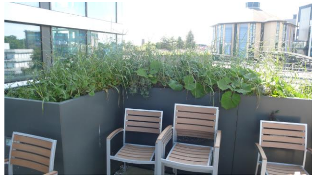
Photo 14: metal planters on the accesible roof terrace of the Fusion building which were in distinctly poor condition and mostly colonised by weeds
