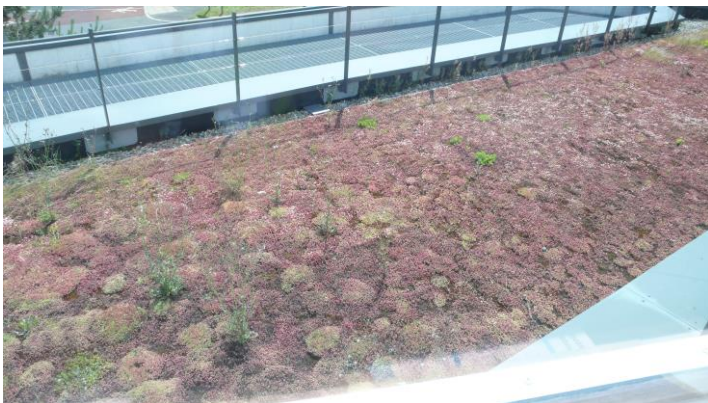
Photo 3: a section of sedum blanket type green roofing on part of the Fusion building which was in good condition with some minor colonisation by weeds
